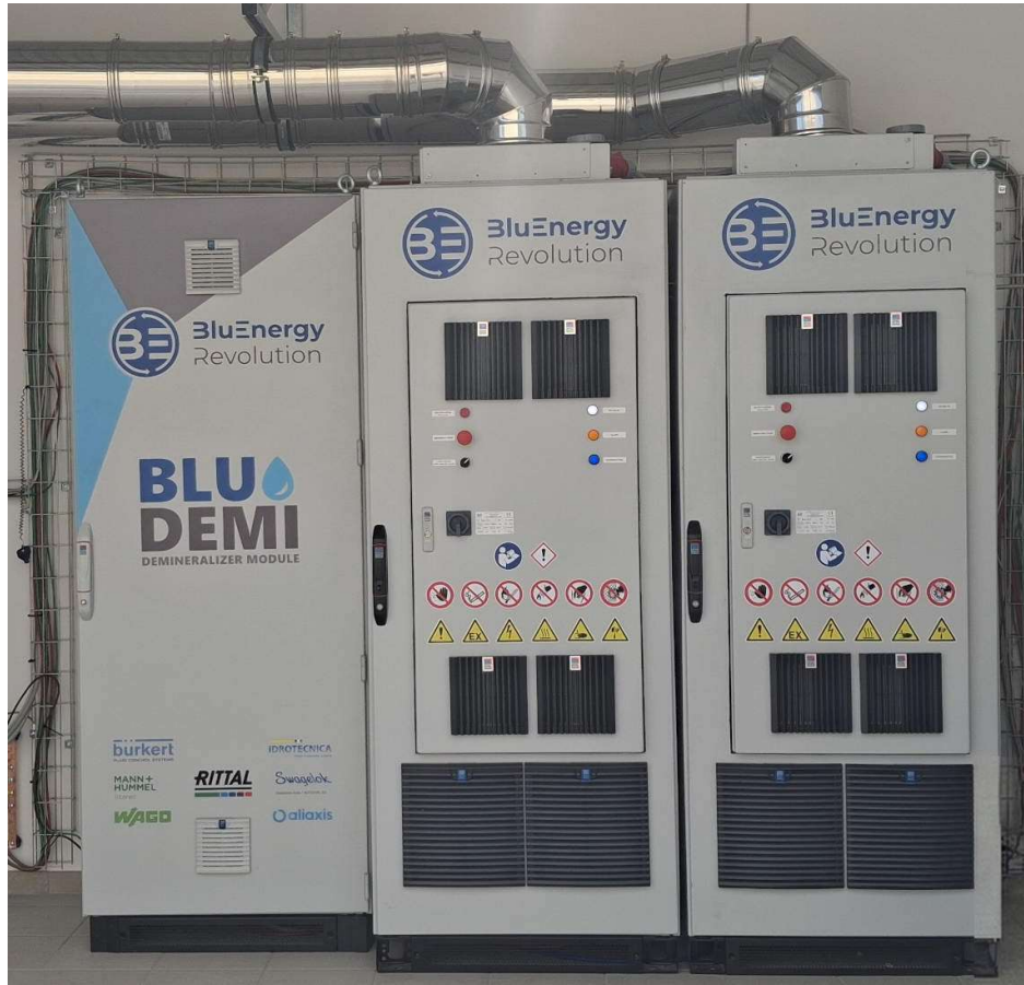
Figure 4-1. A set of 2 MOSE electrolyzers with their water treatment unit.
